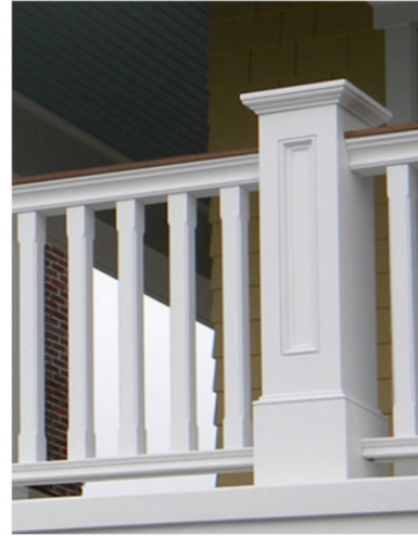
PORCH RAILING: EXISTING TO BE RESTORED AND REPAINTED. NEW RAILINGS TO MATCH EXISTING
